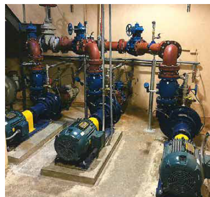
New VFD controlled Influent pumps
