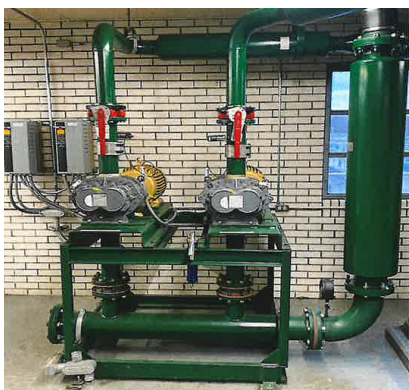
2 New VFD controlled process blowers
