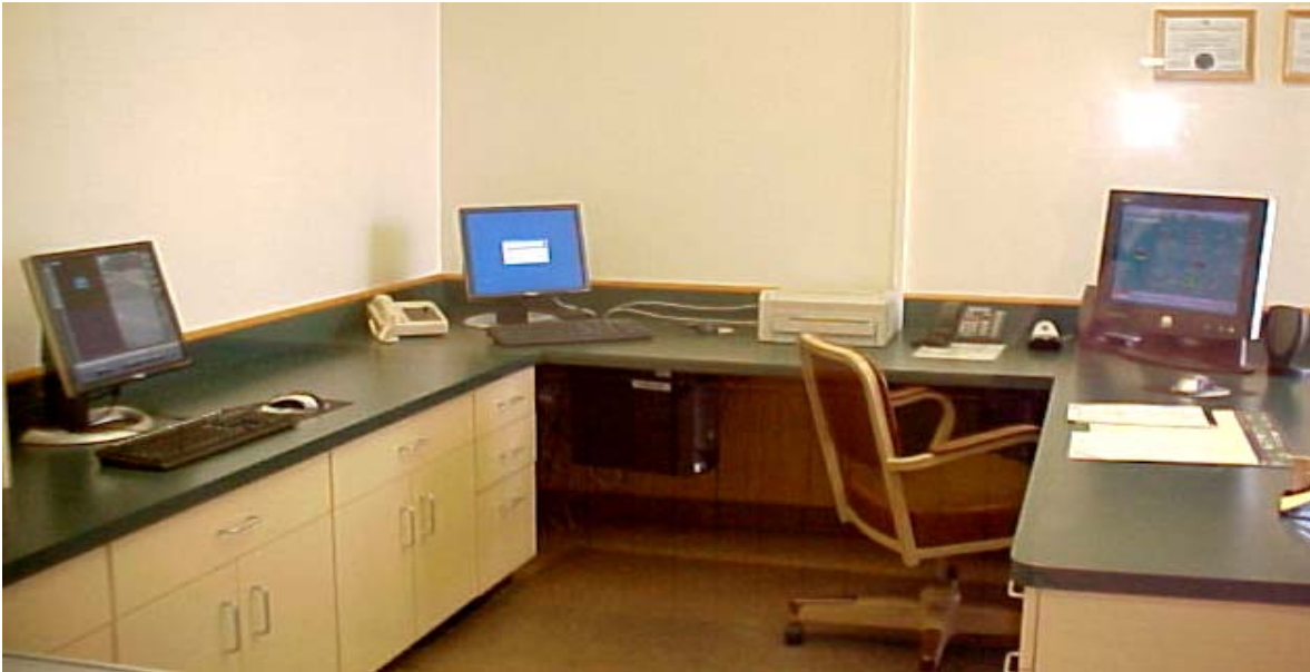
Plant Control Room
