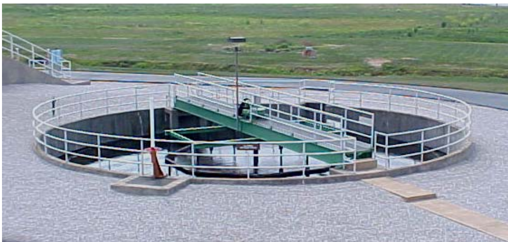
First Stage Settling Tank
