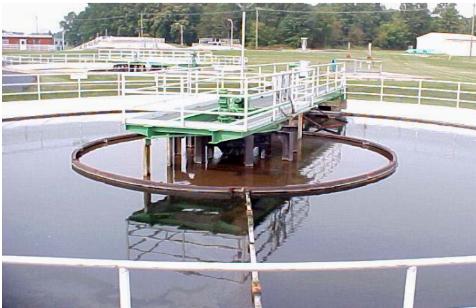
Second Stage Settling Tanks
