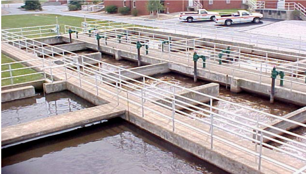
Anoxic Tanks (foreground) Second Stage Aeration Tanks (background)
