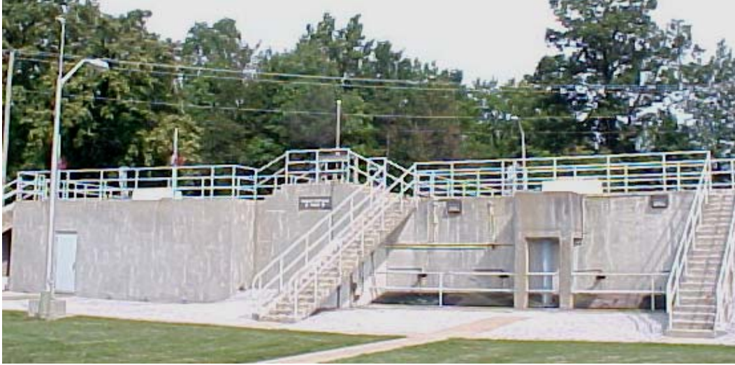
Primary Settling Tanks
